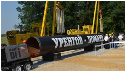
Gas Pipeline, Ukraine. Photo: Dmytro Glazkov . World Bank. Flickr. CC BY-NC-ND 2.0.
